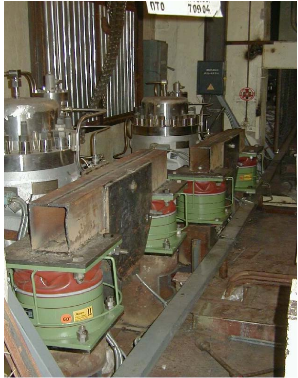
Figure 7. General view of the dampers on the valves 1234 (front) and 1211.
