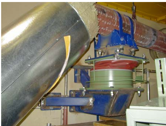
Fig. 8 VES damper at the RL76 in RB LO2 (damper's piston at the piping, housing at the RB wall)
