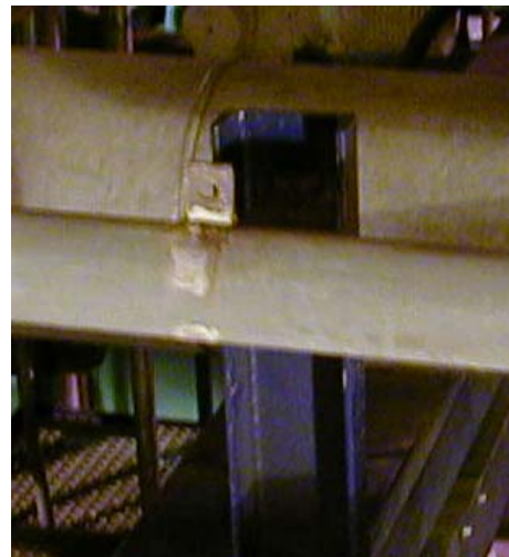
b) fatigue collapse of elastic vibration support
