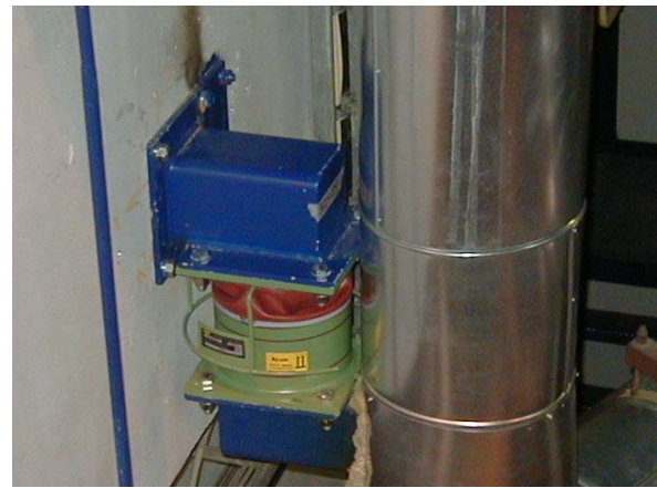
Fig. 11 VRD damper at RA10 line in Deaerator Building (damper's housing at the piping, piston at the vertical wall)
