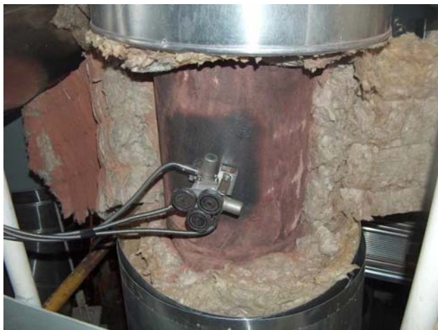
Fig. 2 Example of piping supports degradation due to vibration:
