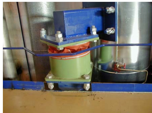
Fig. 9 VD damper at the RA11 in Turbine Hall (damper's piston at the piping, housing at the TH horizontal floor)
