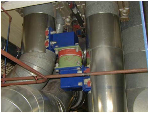
Fig. 10 Connection by VD damper of two RA lines with different dynamic properties.
