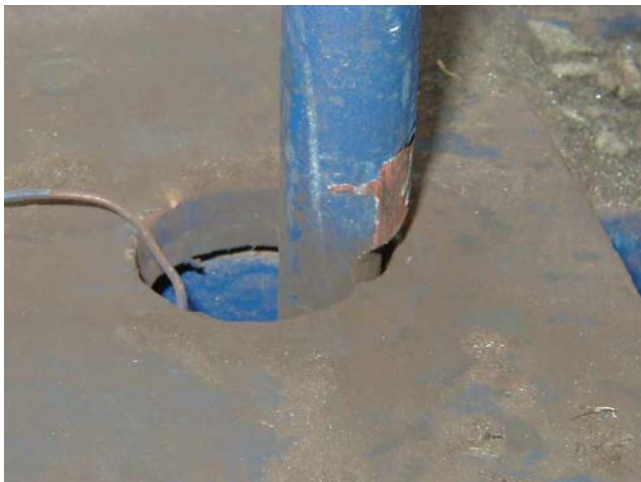
a) wear of the rod hanger
